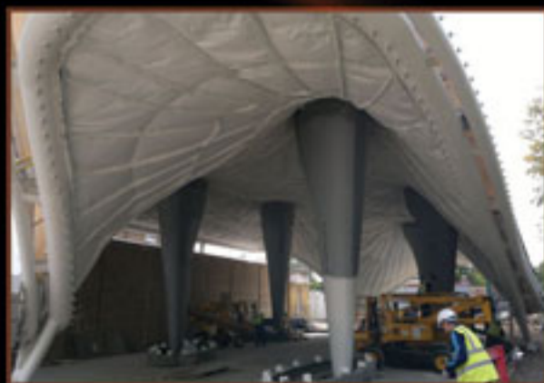
Bespoke Application Fire Protection Serpentine Sackler Gallery UK
